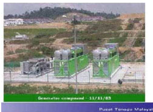
Fig. 7. THS bioenergy plant
