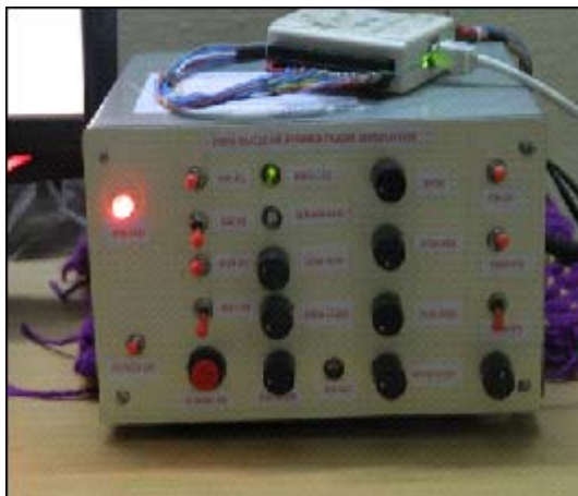
Fig. 9. Indication of power mode in control panel
