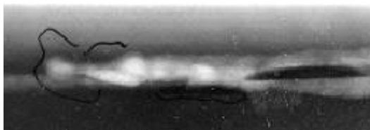
Fig. 3. Radiographs for weld cracks
